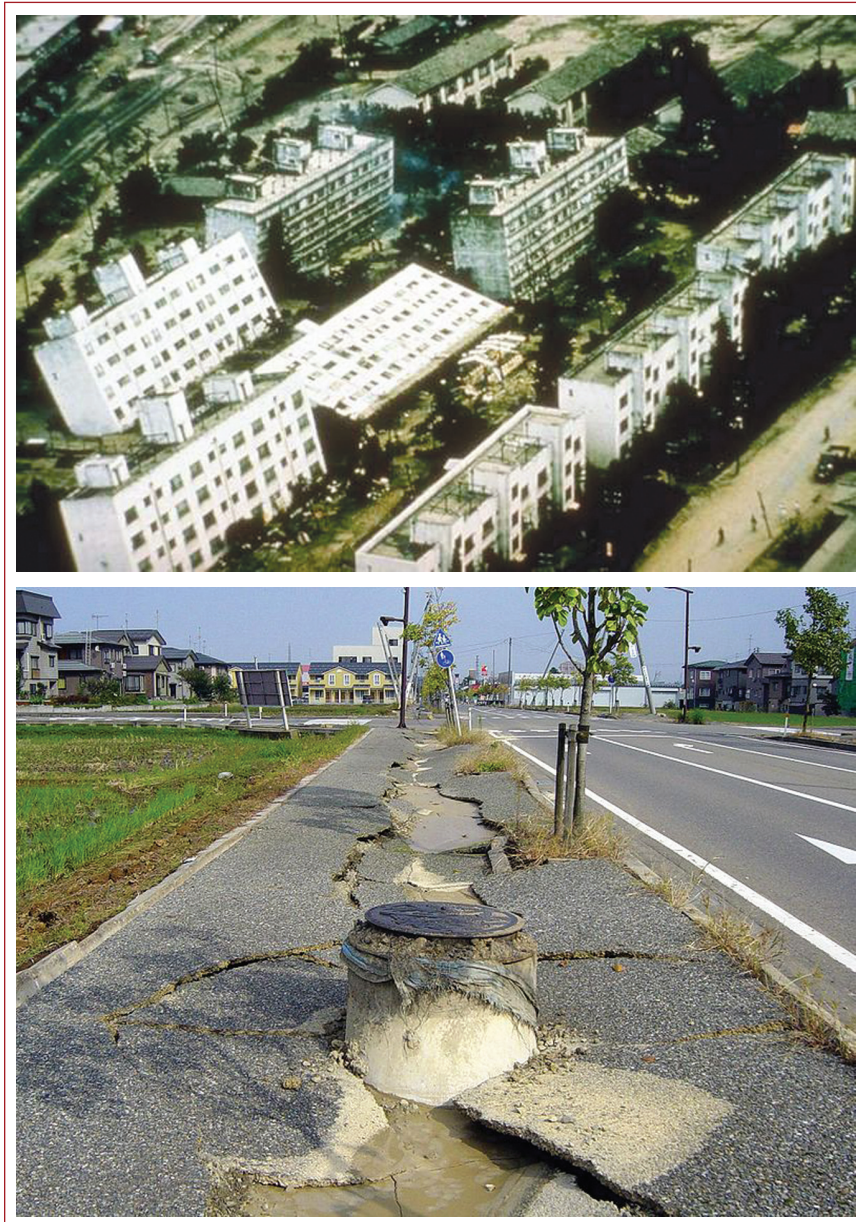
Figure 6 Top photo shows liquefaction-induced settlement of apartment buildings in the 1964 earthquake in Nigata, Japan (photo courtesy of the University of Washington). The bottom photo shows one of many manholes that floated to the surface as a result of soil liquefaction caused by the 2004 Chuetsu earthquake near Nigata, Japan (photo courtesy of Wikimedia Commons).
