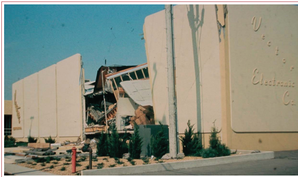
Figure 16 Collapse of a tilt-up building in the 1971 San Fernando earthquake (photo by P. Yaney).
