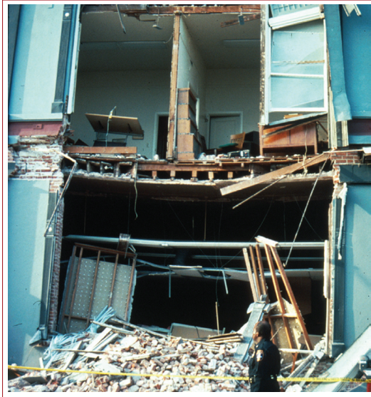
Figure 20 Failure of an unreinforced masonry wall in a building in Santa Cruz, California, in the 1989 Loma Prieta earthquake.
