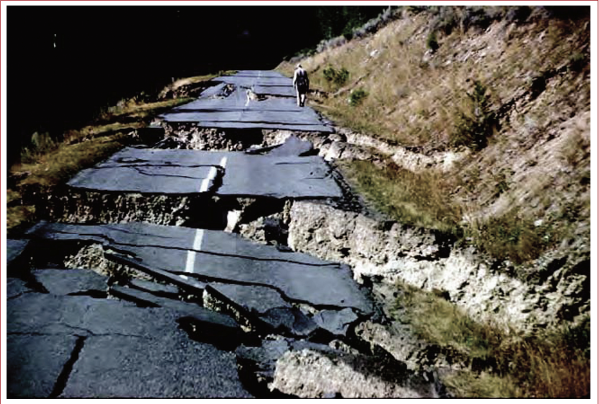
Figure 7 Lateral spreading damage to highway pavement near Yellowstone Park resulting from the 1959 Hegben Lake earthquake (photo courtesy of the USGS).
