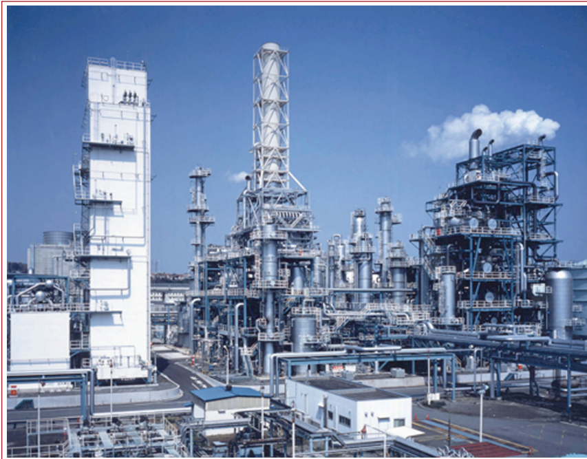
Figure 26 Structures commonly found in petroleum refineries and chemical plants.
