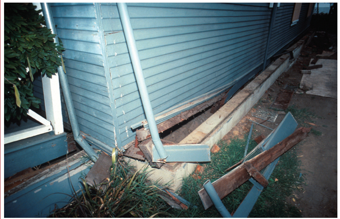
Figure 17 Houses in Watsonville, California, that fell off their foundations in the 1989 Loma Prieta earthquake.
