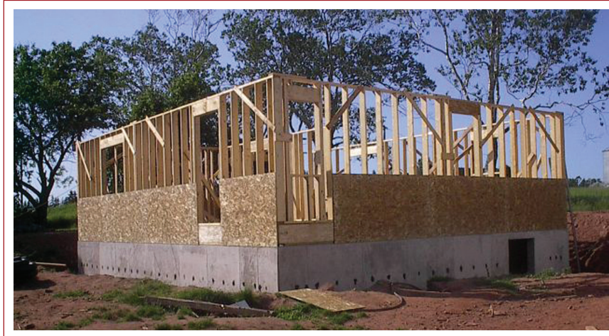
Figure 21 Wood studs and structural panel sheathing of typical wood frame bearing wall construction.
